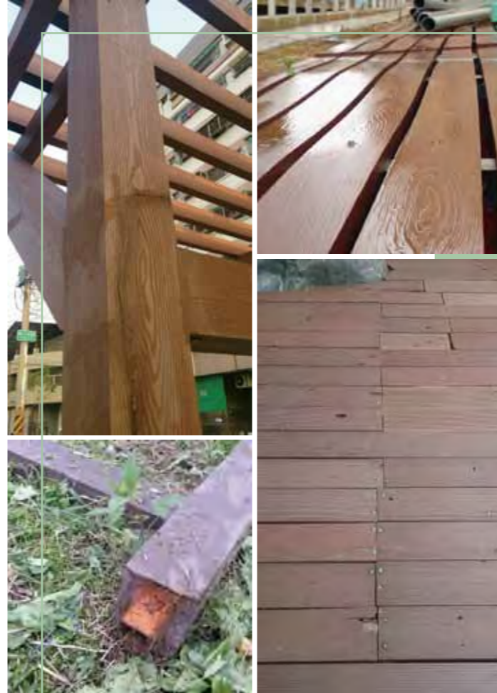
他牌塑木安裝案例 Installation defects from other brands of WPC
